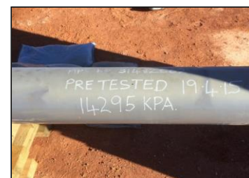
GripTight Testing 12m lengths prior to being installed under a road crossing
