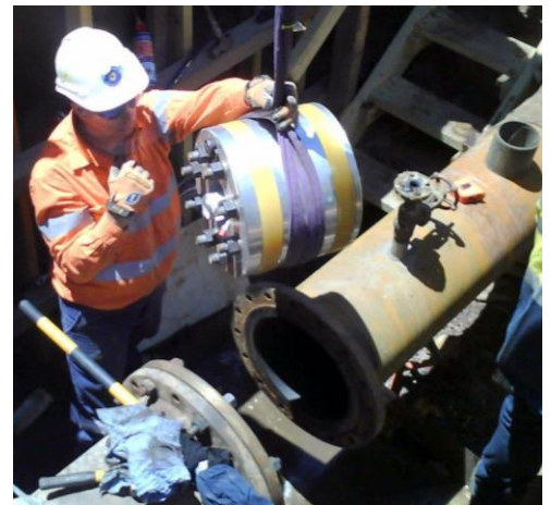
Installing the plug past the 2” branch to Isolate and cold cut the pipe.
