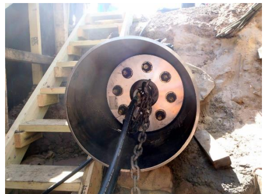
DBB Plug being used to Isolate the line and create a safe area to carry out hot work.
