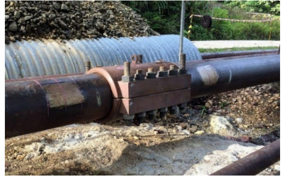
PIPELINE WITH REPAIR CLAMP BUT NOW LEAKING FROM THE SEALS.
