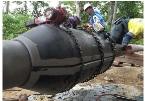
LEAK SEALED AND RAMFILL SLEEVE FITTED READY FOR WELDING.
