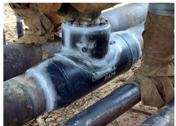
RAMFILL SLEEVE FULLY INSTALLED: WELDED, NDT INSPECTED & FILLED WITH RAM LIQUID EPOXY.
