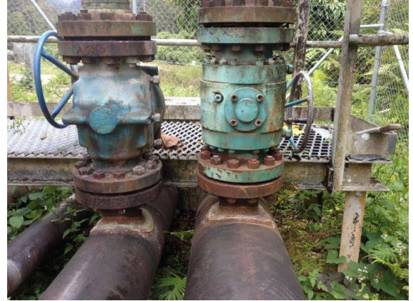
INTERNAL EROSION CAUSED BY SAND
