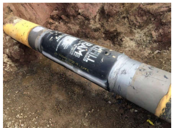
RAMFILL SLEEVE FULLY INSTALLED: WELDED, NDT INSPECTED & FILLED WITH RAM LIQUID EPOXY.
