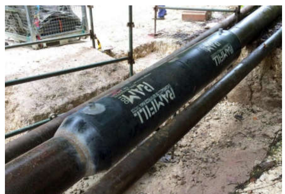
RAMFILL SLEEVE FULLY INSTALLED: WELDED, NDT INSPECTED & FILLED WITH RAM LIQUID EPOXY.
